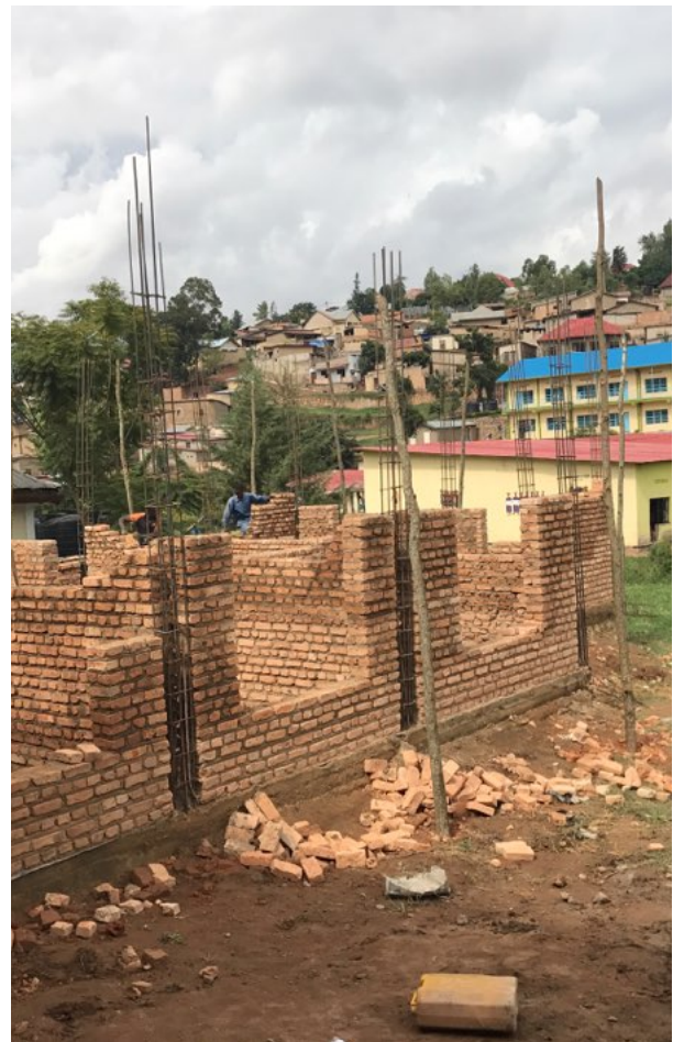
These are the walls for the Teacher Training College, the school is in the background with the blue roof.
